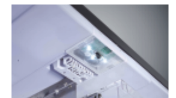
Interior LED light
